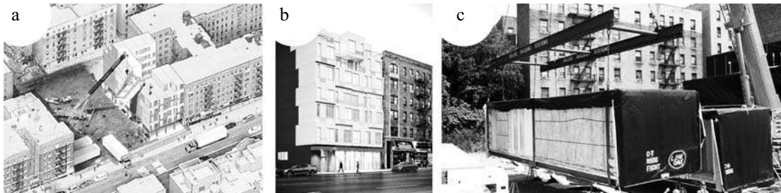
Fig. 2. Method of mounting modules from the adjacent area using a crane (a); appearance of the external facade and volume (b); unloading of the assembled modules at the construction site in New York, USA (C) (The Stack Modular Housing in Manhattan / Gluck + [Electronic resource] // ArchDaily. – 2020. – Resource access mode: https://www.archdaily.com/943491/the-stack-modular-housing-in-manhattan-gluck-plus?ad_source=search&ad_medium=search_result_all )
