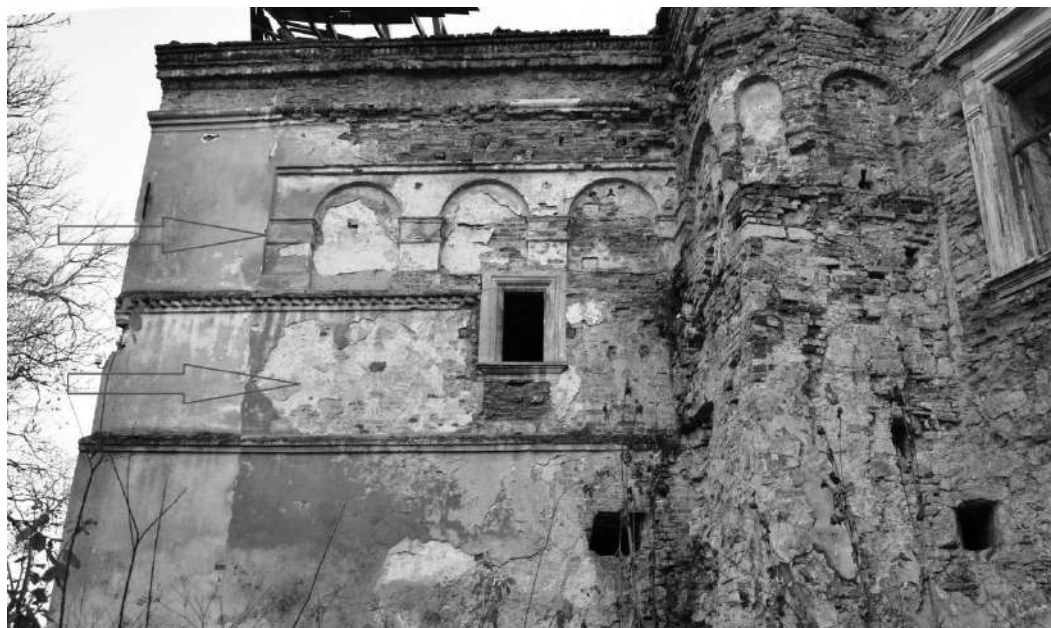
Fig. 4. The north wall of the corner tower of the Pomoryany castle. The places where the polychrome paintings preserved are indicated with arrows
