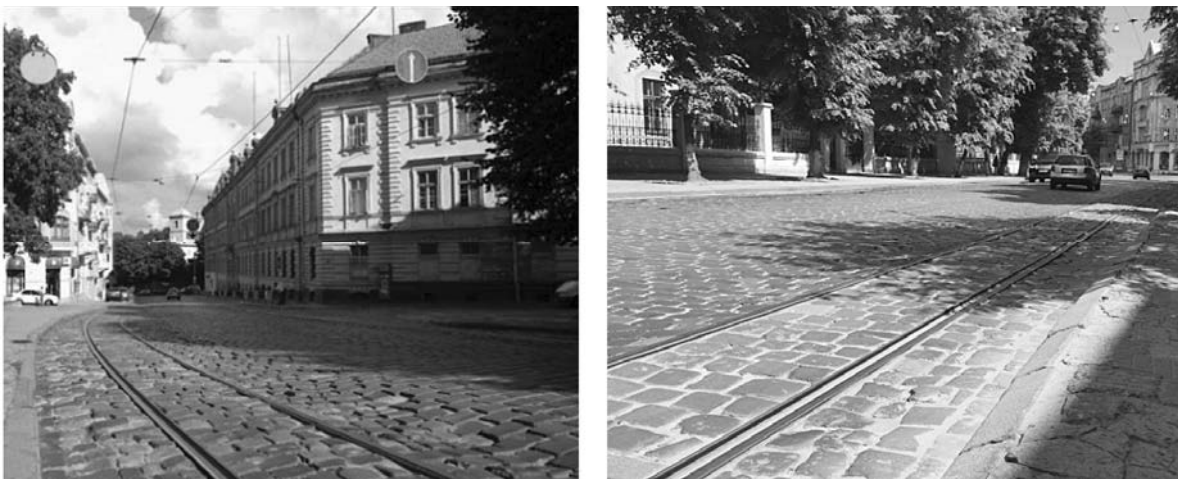
Fig. 2. The present condition of the road surface from the pavement side, Bandera street, 2018, [9]
