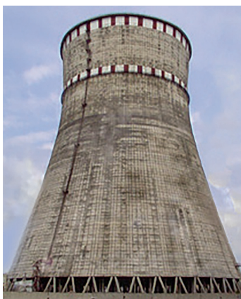
Figure 1. Natural-draft RC cooling tower, height H = 150 m, wetted area 10,000 m 2
